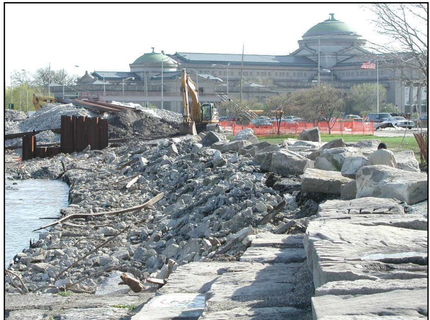
Beginning construction for traffic lights at 57th Street and Lake Shore Drive, 2001
